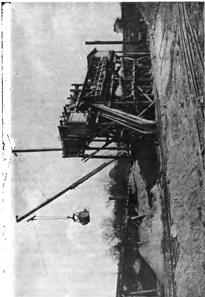
PLATE 170.—Central Concrete Mixing Plant of Large Capacity. Sand and stone raised to bins by derrick with “grab” bucket. Concrete mixed in tilting mixer which discharged into bottom-dumping buckets hauled to site of work on cars.
